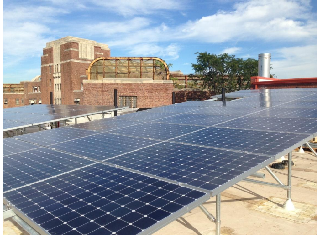
Rooftop solar installation at CAMBA Gardens
